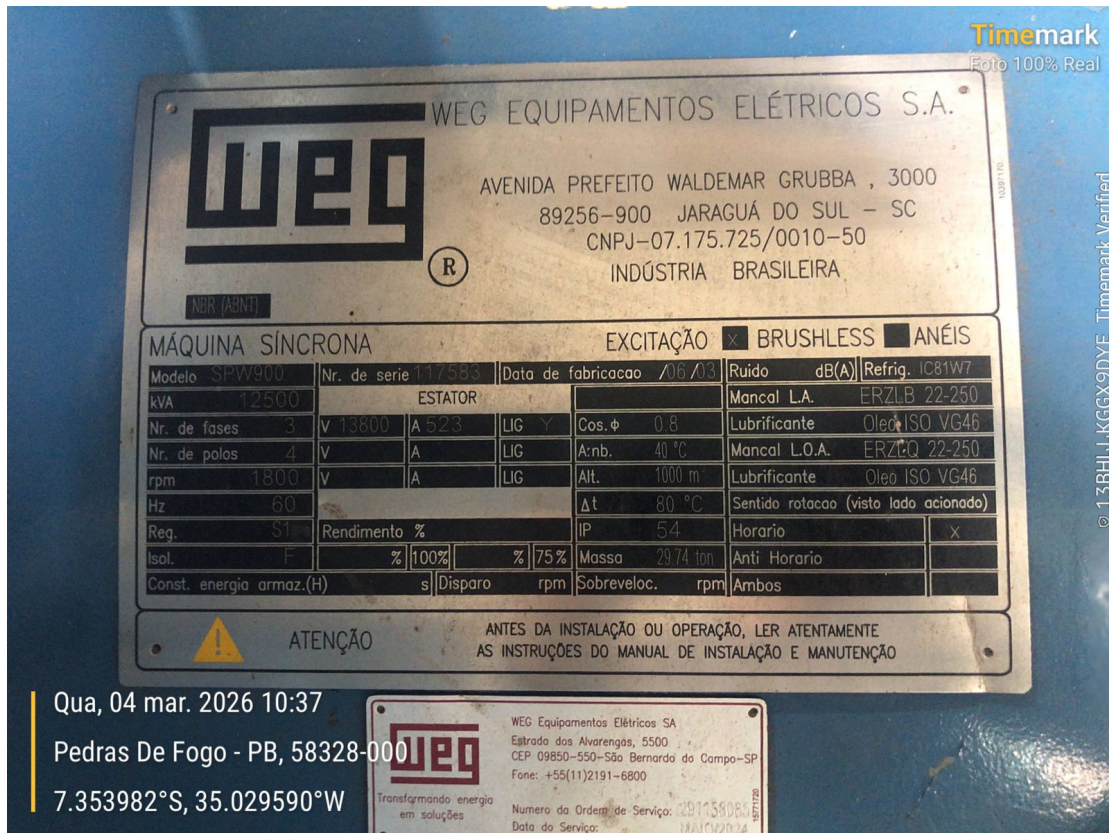
Alternator/ Generator UG 8
