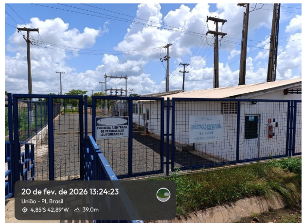
10 MVA Step-up Substation
