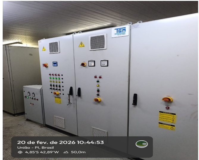
TGM Turbine Panel – UG5
