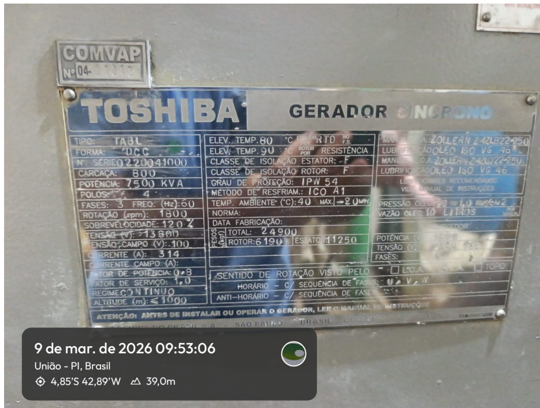
Alternator/ Generator UG 1
