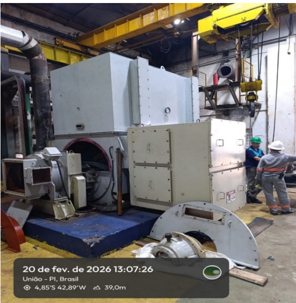
Alternator/ Generator UG 1
