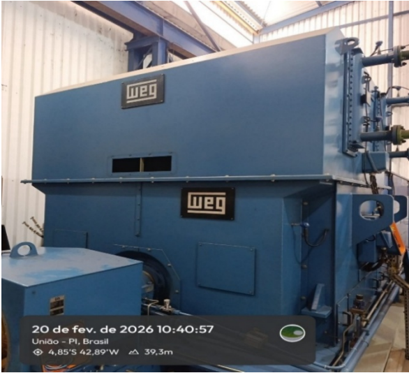
Alternator/ Generator UG 5
