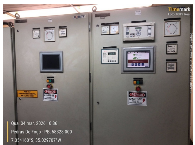
Protection and Control Panels
