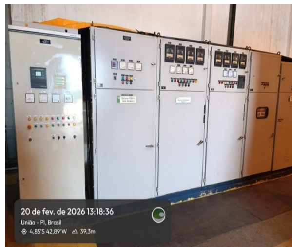
Generator Excitation & Protection System – UG4
