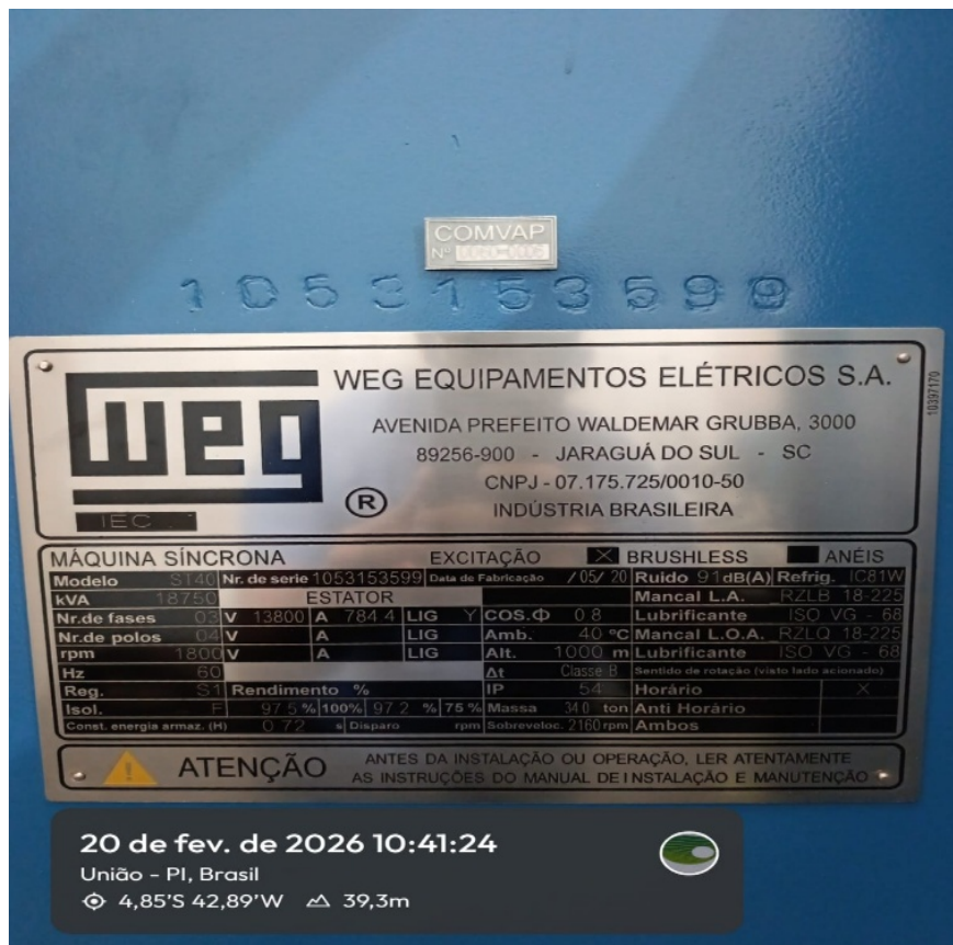
Alternator/ Generator UG 5
