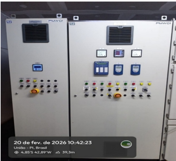
Generator Excitation & Protection System – UG5
