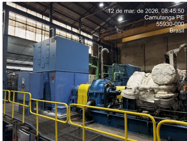
Alternator/ Generator UG 2
