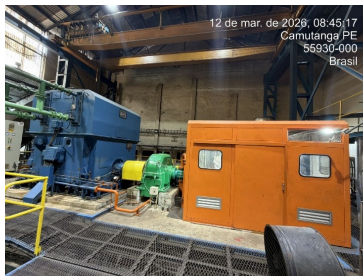
Alternator/ Generator UG 3
