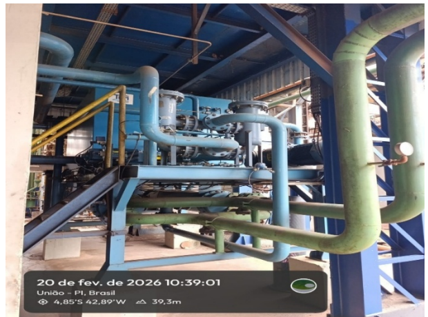
Generator Lubrication System – UG5
