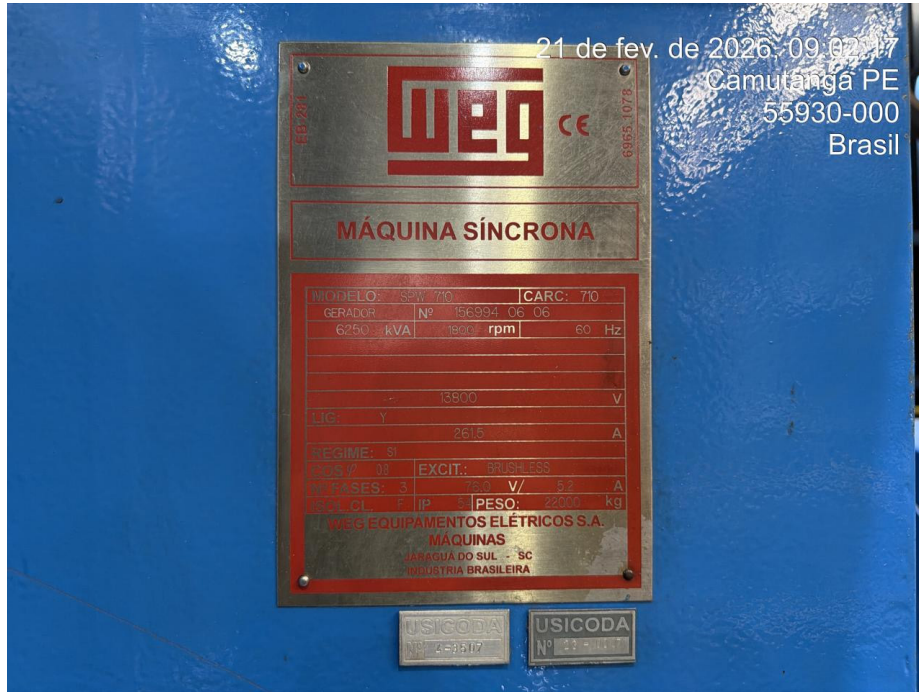
Alternator/ Generator UG 1
