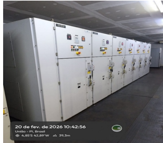
Medium Voltage Distribution Panels
