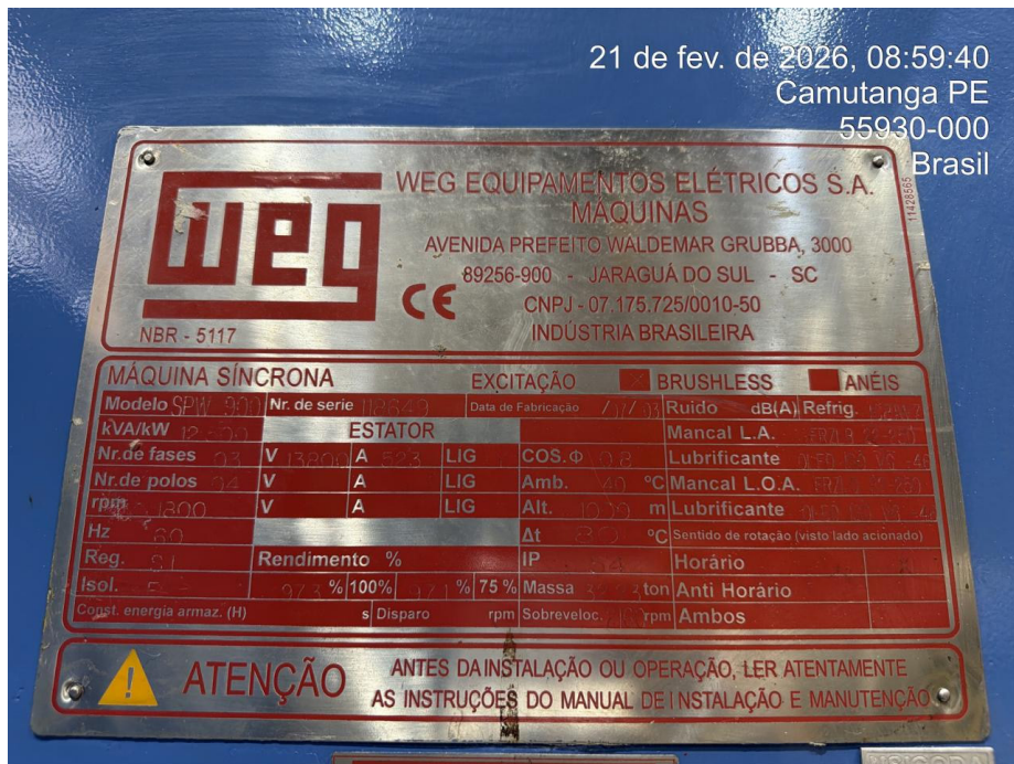
Alternator/ Generator UG 2
