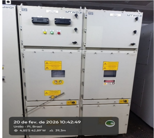
Generator Circuit Breaker Panel – UG5
