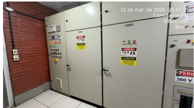
Medium Voltage Panel
