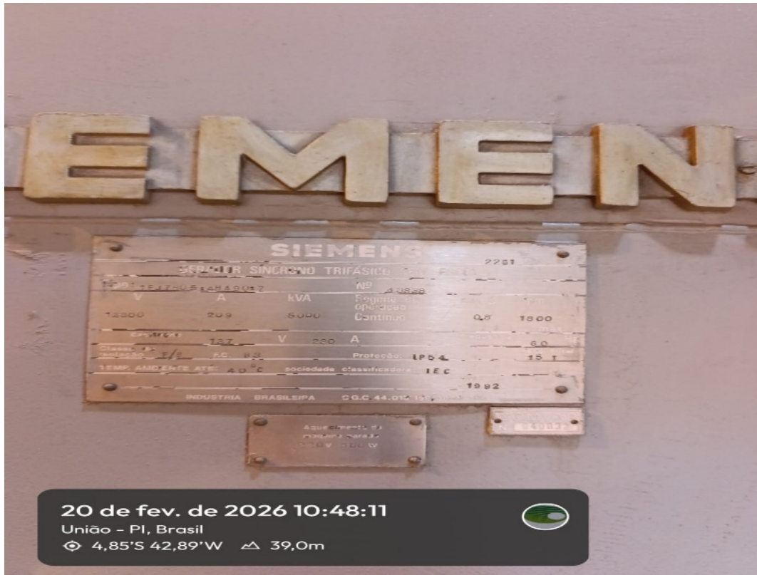
Alternator/ Generator UG 4
