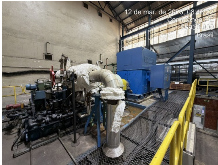
Alternator/ Generator UG 1
