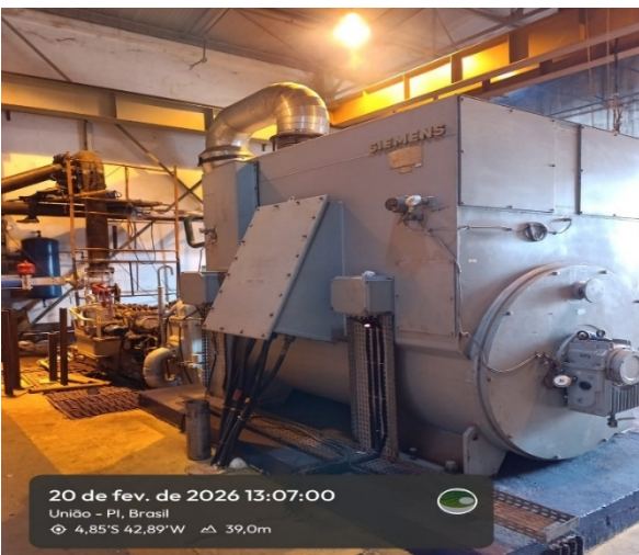
Alternator/ Generator UG 4
